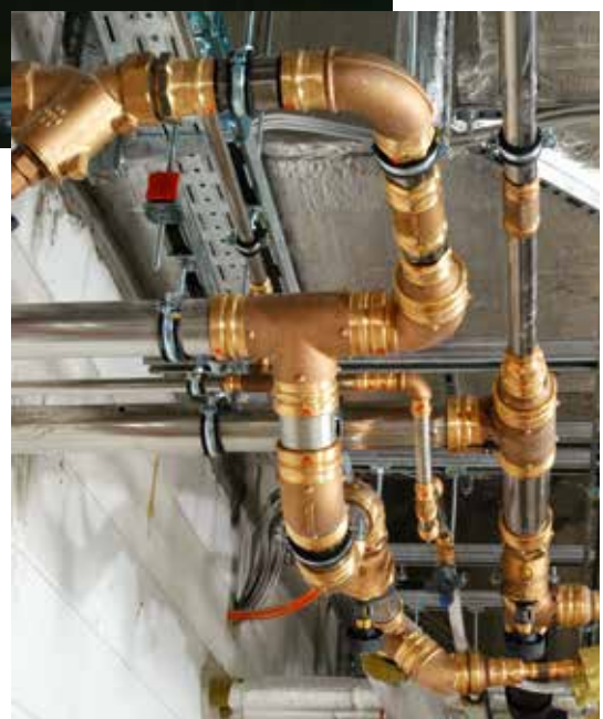
A total of 8 kilometres of Sanpress stainless steel piping was installed for the main drinking water distribution system.
